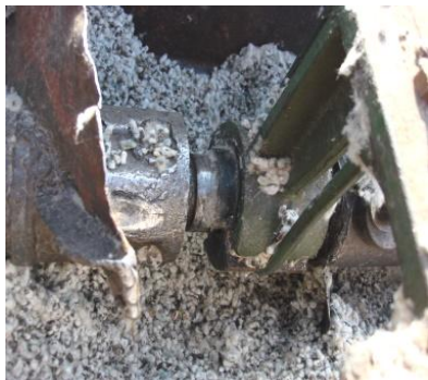
Figure 13. Sliding bearing installed in the friction unit of screw conveyor.
